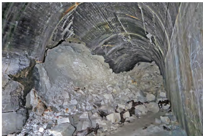
Demolition rubble at the site of the north portal. Photo Clive Penfold
